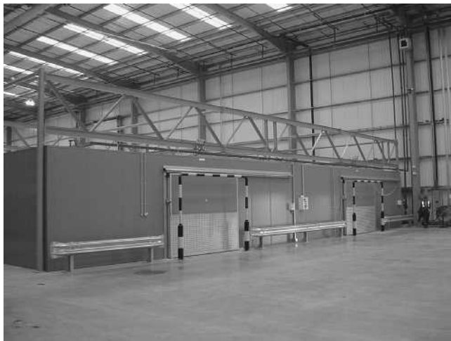
Figure 17.8 Refrigerated compartment within a warehouse for a range of frozen and chilled products (Star Refrigeration)
