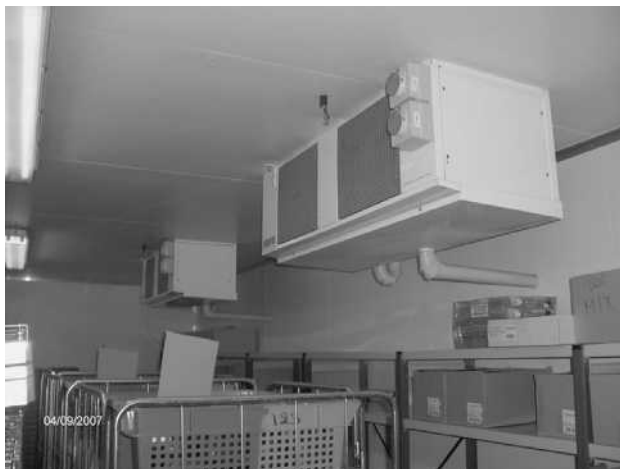
Figure 15.8 Ceiling-mounted coolers (Michael Boast)
