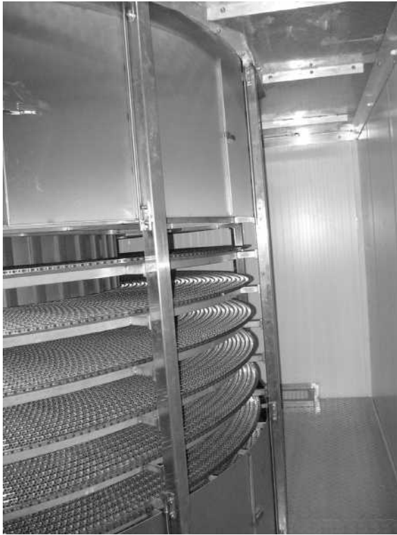
Figure 14.2 View of spiral freezer (Star Refrigeration)
