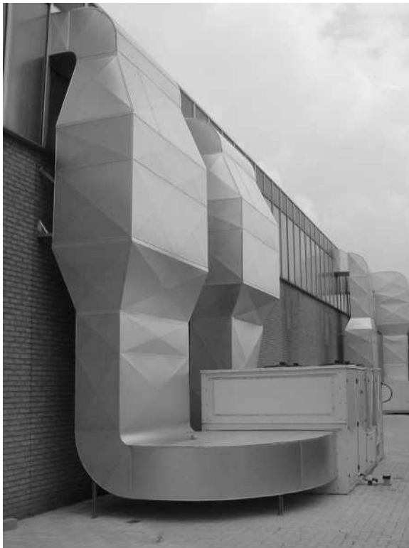
Figure 25.3 Air-handling units providing air conditioning for production plant, total installed capacity 145 kW (Johnson Controls)
