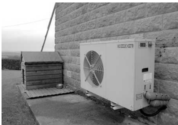
Figure 27.4 Wall mounted ASHP delivering 8 kW heating to a farmhouse in Appleton le street, North Yorkshire (HeatKing)
